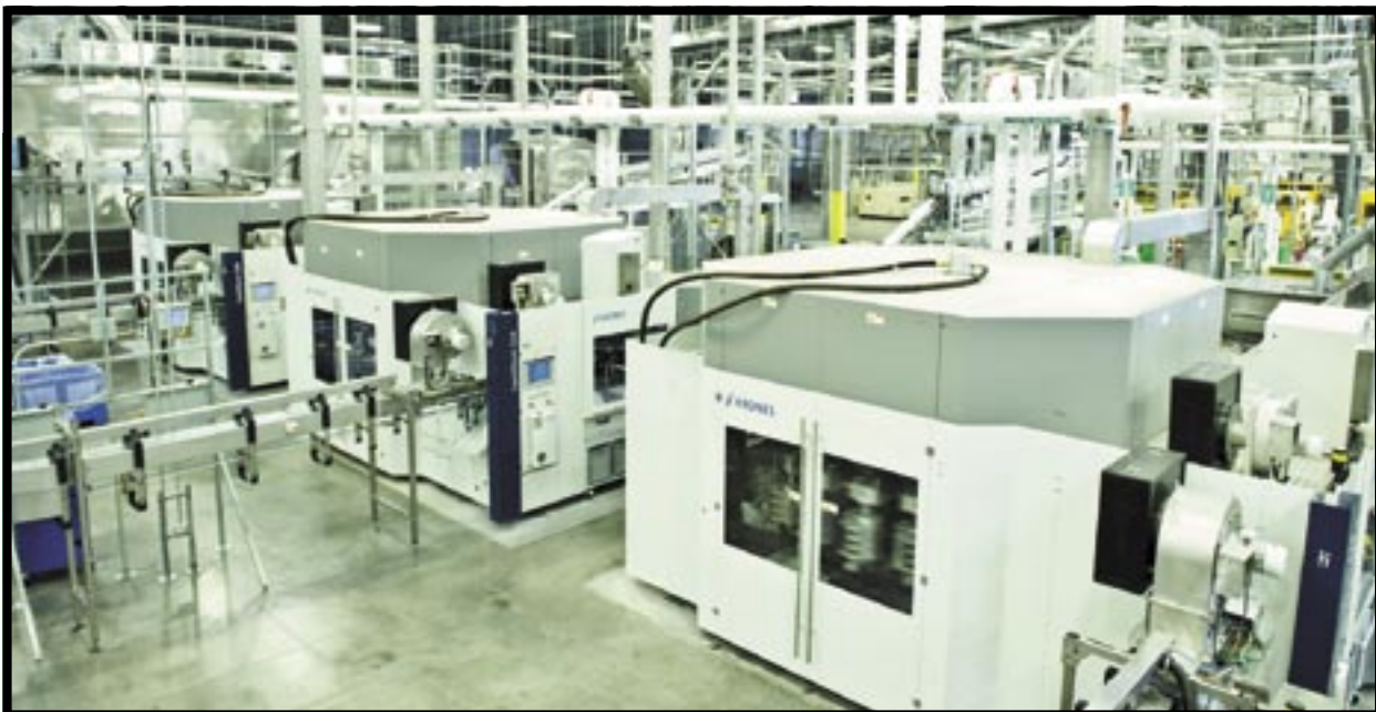
The new facility at Dallas in Texas likewise received two 72,000-bph PT lines in a twin configuration.
