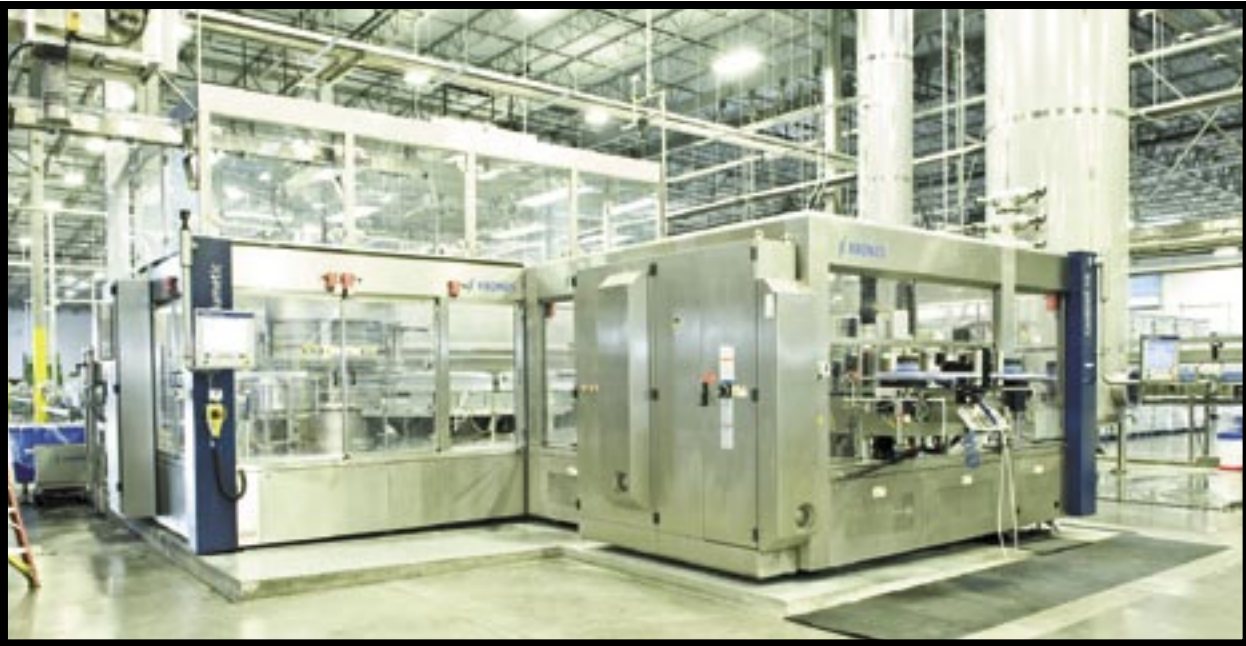
The labeller/filler BLOC, comprising a Contiroll HS and a Sensometric VOG-PET , prelabels the empty containers before they are filled.
