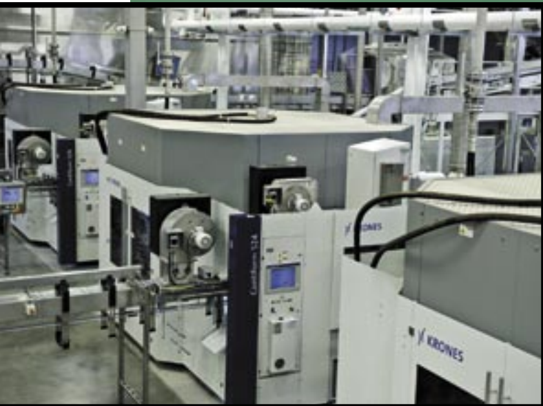
Three Contiform S24 blow-moulders (each rated at 43,200 containers an hour) supply two labeller/filler BLOCs, each in their turn producing between 64,800 and 72,000 bottles per hour.
